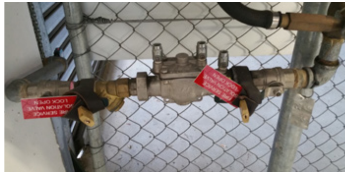
LOW HAZARD DEVICE ON A FIRE SERVICE
