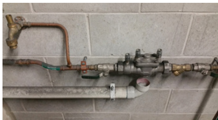
HIGH HAZARD DEVICE IN A BASEMENT
